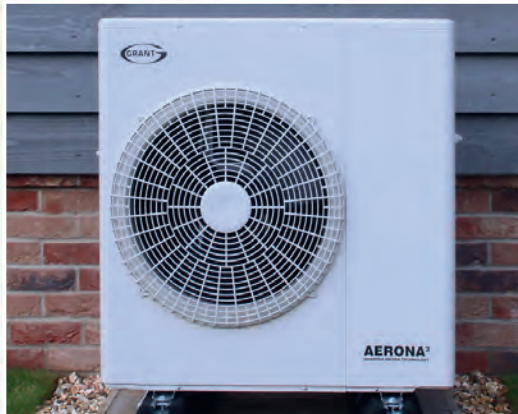
Air Source Heat Pumps / Electric Storage Heaters
