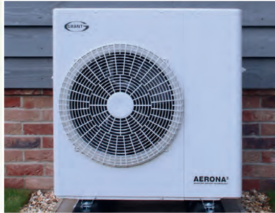
Air Source Heat Pumps / Electric Storage Heaters
